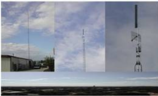
Base Station for Bandera Site
